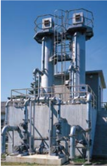
Trichloroethylene removal system
