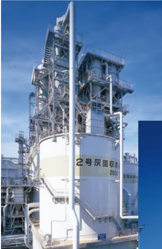
Ash Handling System
