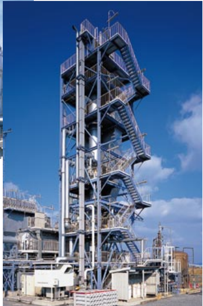
RDF (Refuse Derived Fuel) boiler flue gas treatment system
