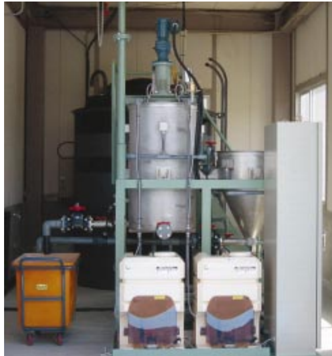
実証試験設備 Equipment of demonstration test
