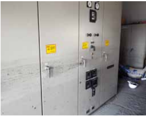
図6 受変電設備浸水 Flooded electric incoming and substation facilities
