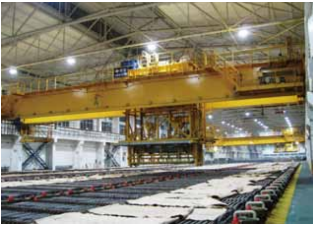
図2 銅電解用天井クレーン Overhead crane for copper electrolysis facility
